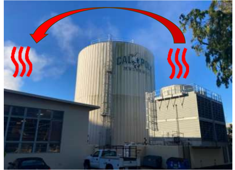
Cal Poly's Central Plant Source: Chad Worth
